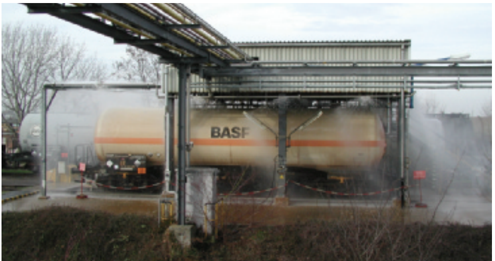
Figure 24 The ammonia loading area. The complete RTC is covered with water from the hydro-shields
