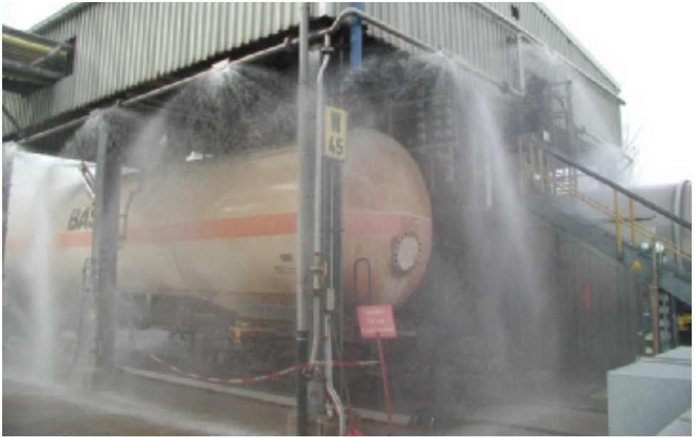
Figure 23 The water curtain system in action. The sprayed water builds a closed curtain
